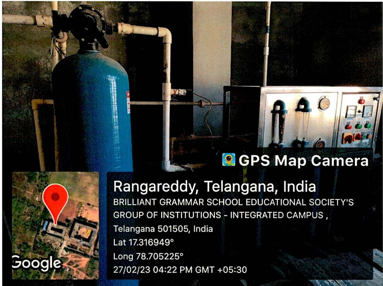
RO water plant.
